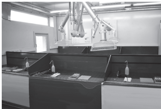
Figure 7.3. Laboratory equipped with extraction systems suitable for handling the volatile emissions of adhesives and other chemical used in the bonding process.
